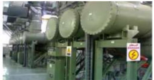
Sabik Gas Jubail GIS Substation
