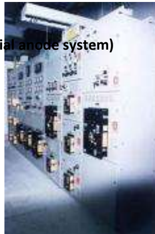
LV switchgear serving Expec computer center (S. Aramco)
